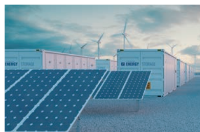
Energy Storage System
